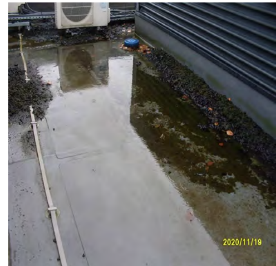
Ponding water and detritus
