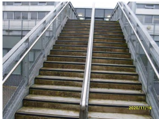
Stair risers requiring cleaning
