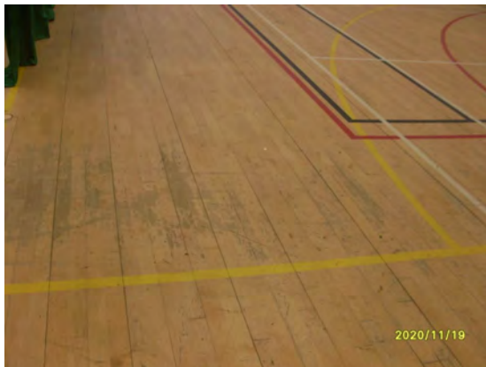
Wear to gym floor
