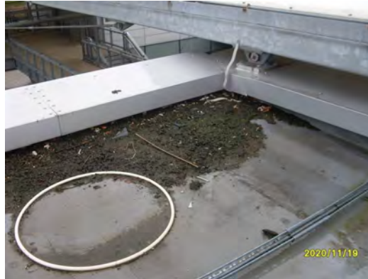
Build-up of detritus
