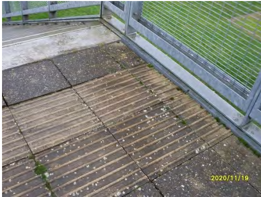
Loose tactile paving at landing
