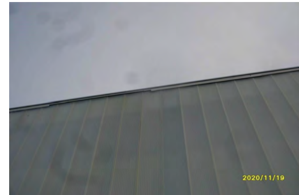
Missing trim to gym cladding
