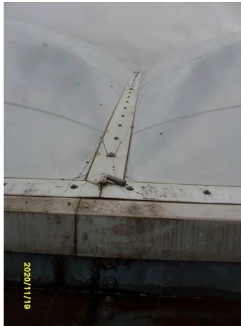
Broken anti-bird wires
