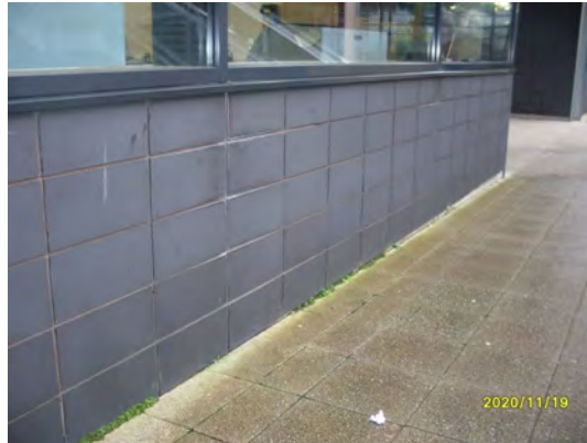
Water run-off and staining to blockwork
